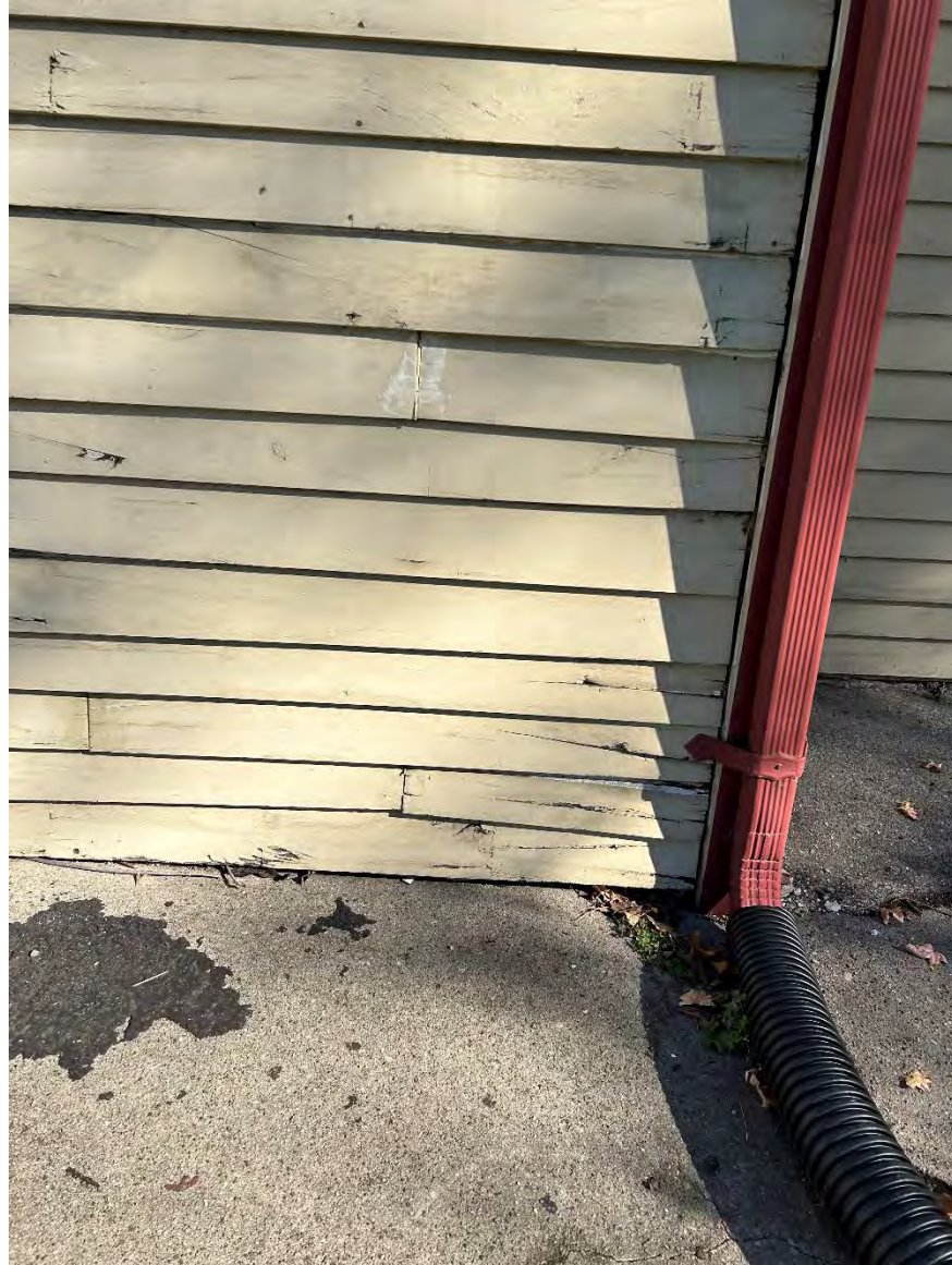
Figure 4: Photo of exterior damage to the addition proposed to be partially demolished.
