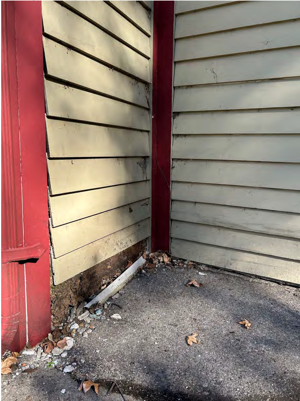
Figure 5: Photo of exterior damage to the addition proposed to be partially demolished.
