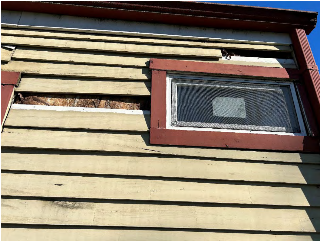
Figure 6: Photo of exterior damage to the addition proposed to be partially demolished.
