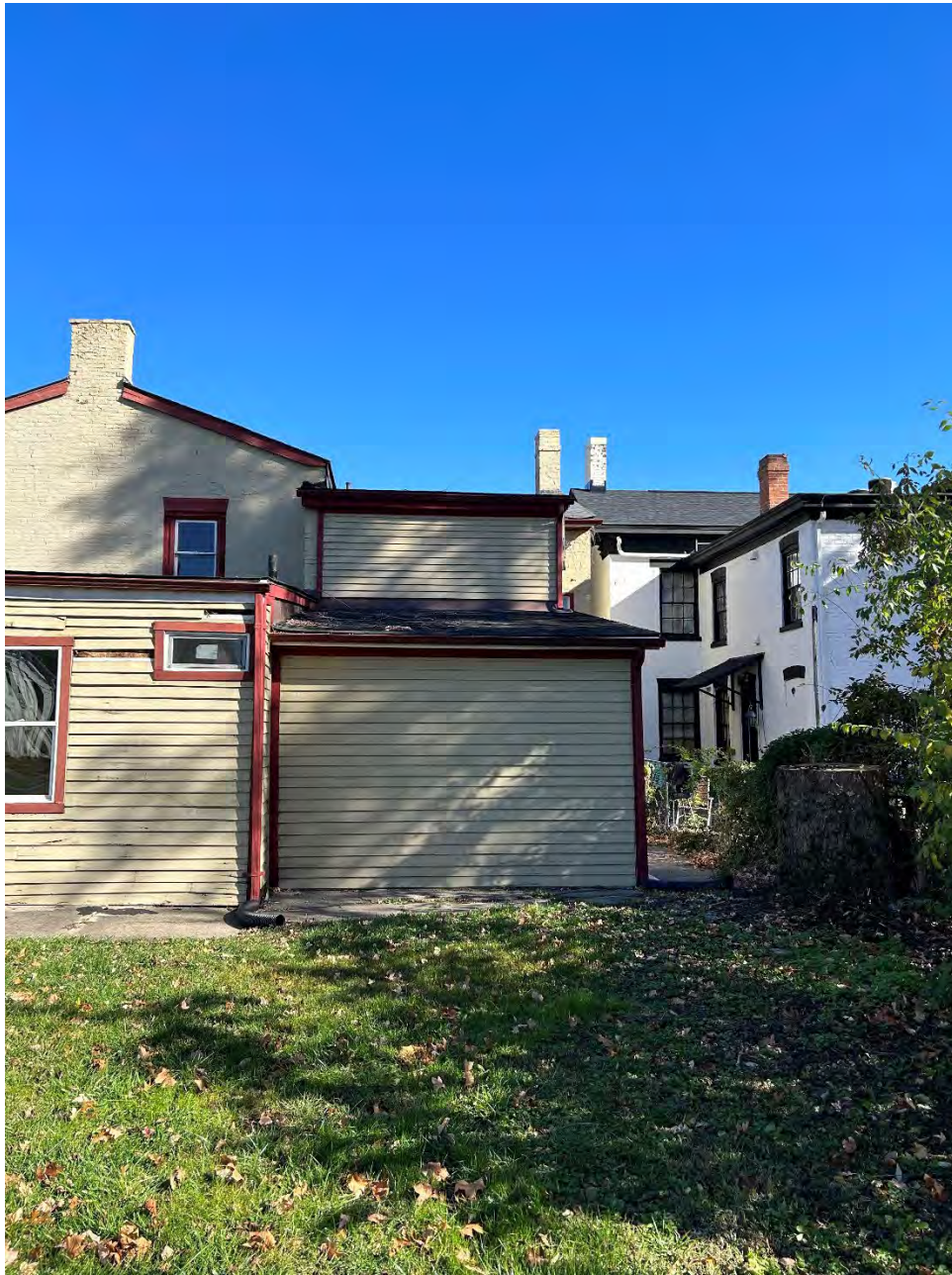
Figure 2: Photo of the exterior of the addition proposed to be completely demolished.
