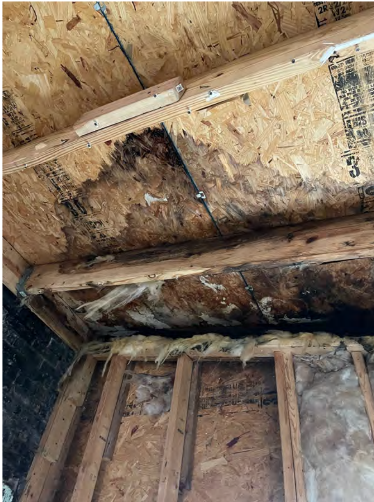
Figure 5: Photo of the interior damage to the addition proposed to be fully demolished.
