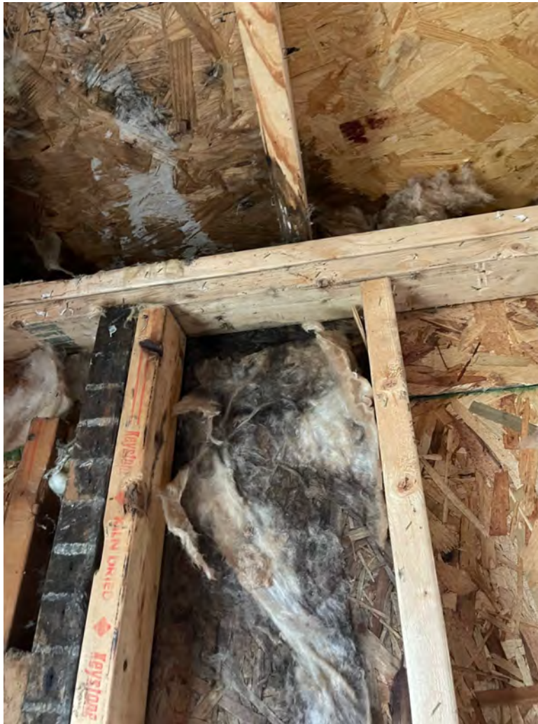
Figure 4: Photo of the interior damage to the addition proposed to be fully demolished.
