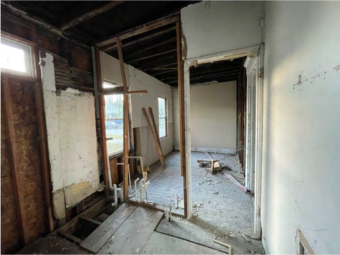
Figure 9: Applicant is proposing to keep the roofline as a covered porch area.
