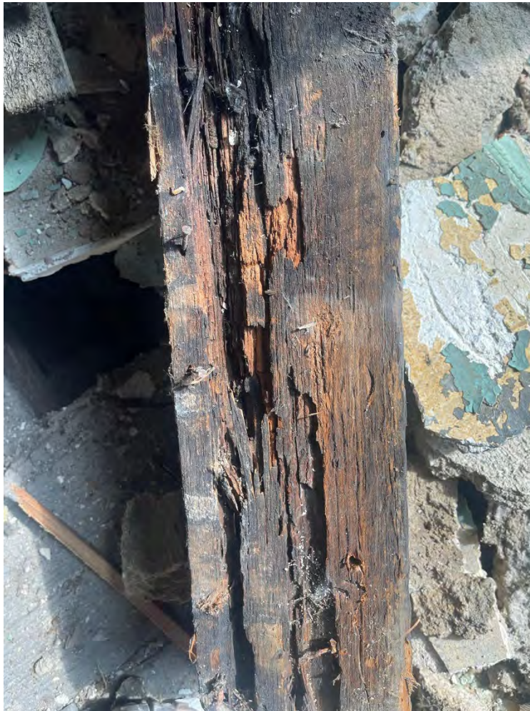
Figure 7: Photo of the interior damage to the addition proposed to be partially demolished.
