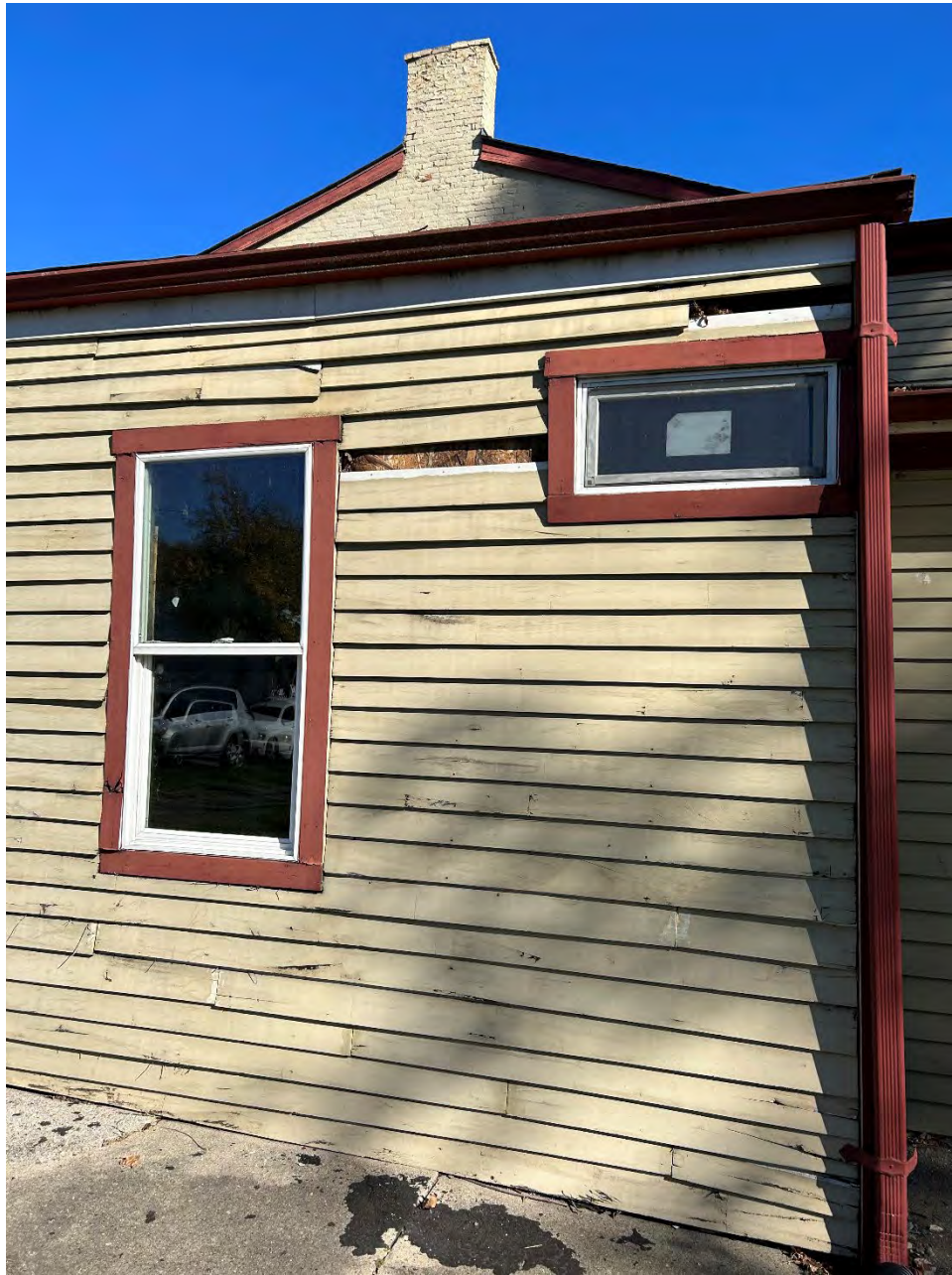
Figure 3: Photo of exterior damage to the addition proposed to be partially demolished.
