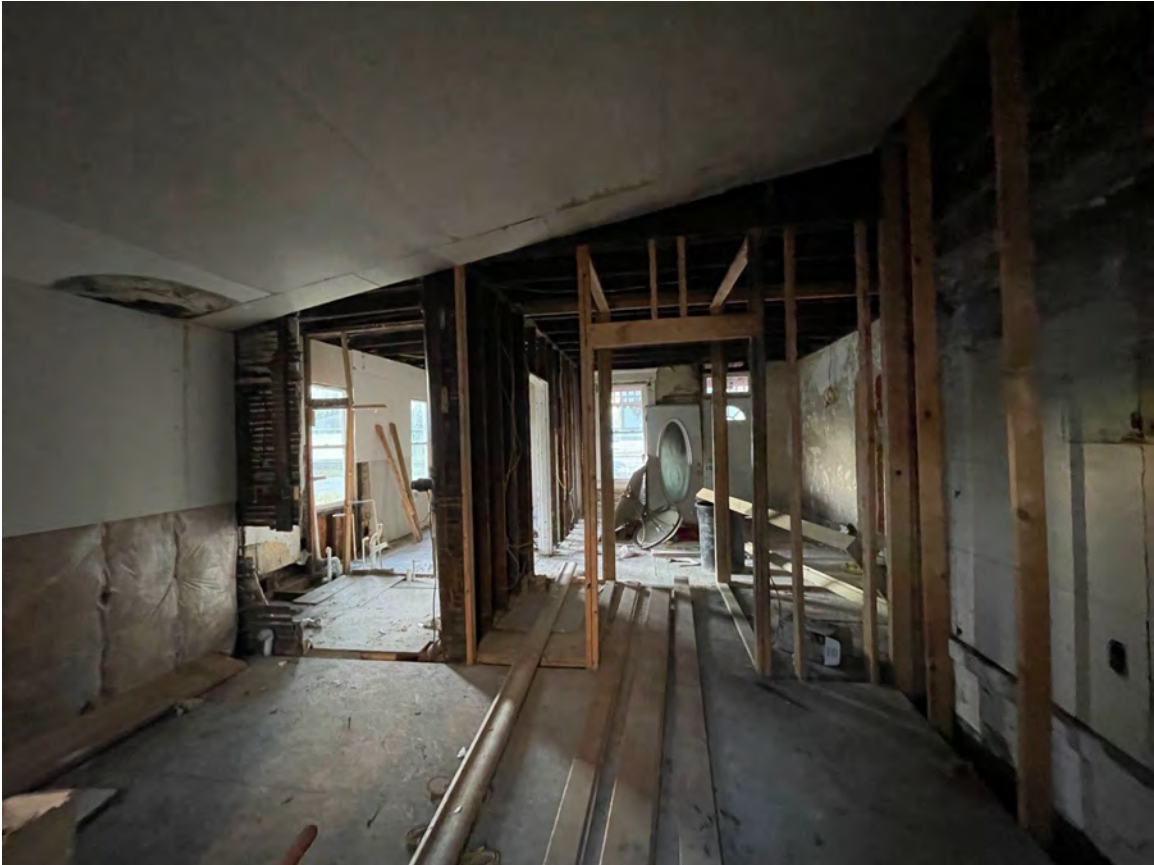
Figure 1: Photo of the interior damage to the addition proposed to be fully demolished.
