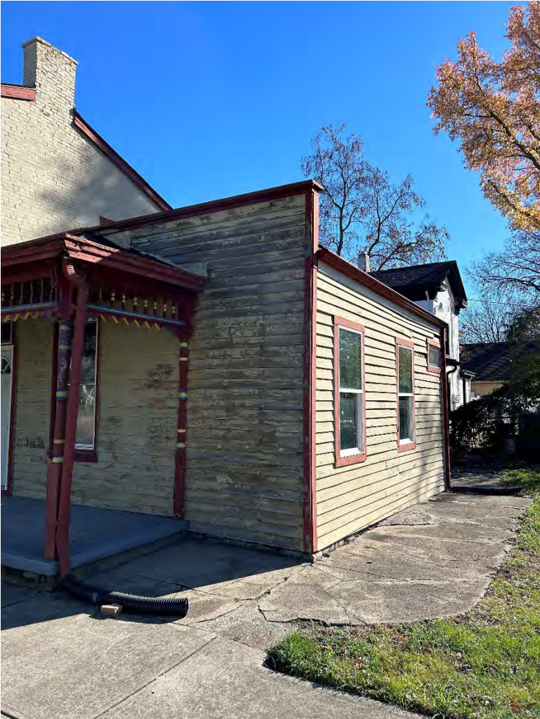
Figure 1: Photo of the exterior of the addition proposed to be partially demolished.
