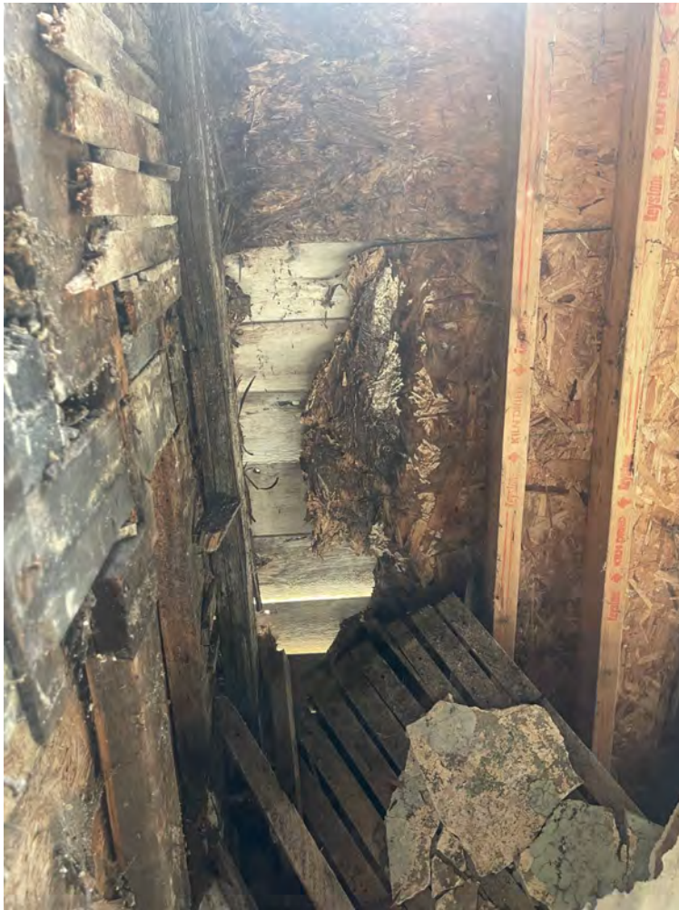
Figure 6: Photo of the interior damage to the addition proposed to be partially demolished.
